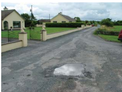
Photo 16: The occasional pothole is evident on road edges and road junctions. Otherwise roads through the village are in very good condition.
