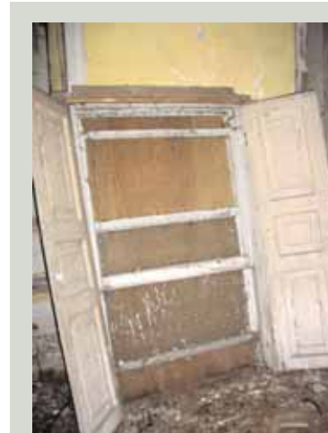
The window frame assemblage should not be removed from the structural opening unless this is necessary. If it must be removed, this should be done immediately prior to repairs being carried out, as otherwise the assemblage could be left vulnerable to damage
