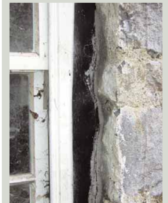
The silicone-based mastic used here is starting to lift in places, just a few years after being applied. As it is black and applied thickly it is more visible than caulking or pointing should be
