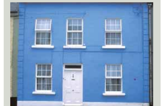
Possibly with the best of intentions, they were taken out and top-hung uPVC casements fitted instead. When closed these appear flat and insubstantial, and when swung open the superficial likeness to traditional windows is lost
