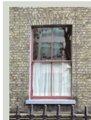
This window was photographed after being carefully cleaned and repainted by the householder
