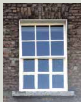
Over-cautious sealing of the putty by painting very far onto the glass can affect the appearance of the window, especially if it is not done consistently
