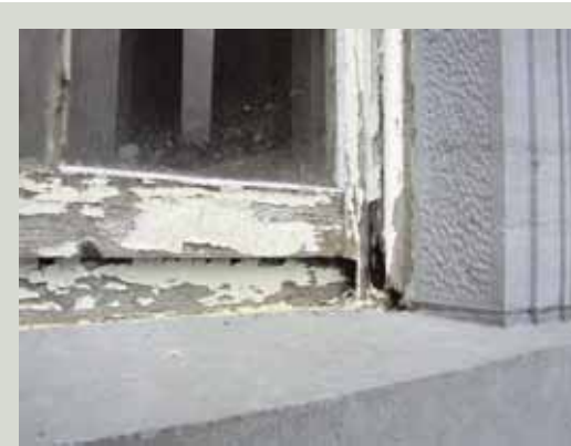
The loss of paint should not be the main guide as to the condition of the timber. Despite years of neglect, this window did not require substantial replacement of timbers. The ends of the box frame and its linings, as the most vulnerable areas, did require new scarfed repairs
