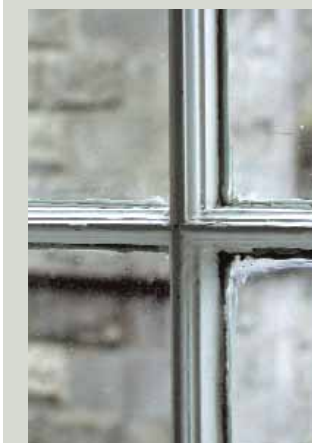
At some stage one of the glazing bars in this sash was repaired (vertical bar, top half of picture). While this kept the sash in use, a standard moulding was used instead of a profile matching the late eighteenth-century original. Small details like this should not be overlooked by those in charge of a repair job
