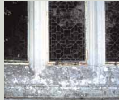
Corrosion at the bottom rail of these casement windows is distorting the metal and damaging the leaded glass. The affected areas will have to be cleaned of rust and dents straightened. It will be necessary to cut out the badly affected metal and patch with accurately profiled new steel
