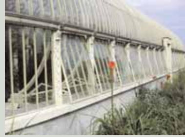
Chemical analysis and performance testing was carried out by the Office of Public Works prior to choosing new paint for the metalwork of the mid nineteenth-century glasshouses at the National Botanic Gardens. It was found that immediate sealing of the metal - within twenty minutes of drying the bare metal - increased the protection that the paint gives by a factor of five
