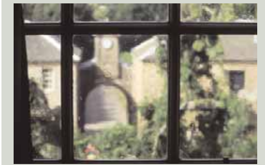
This film contains many bubbles and in general reduces the clarity of the view through the glass
