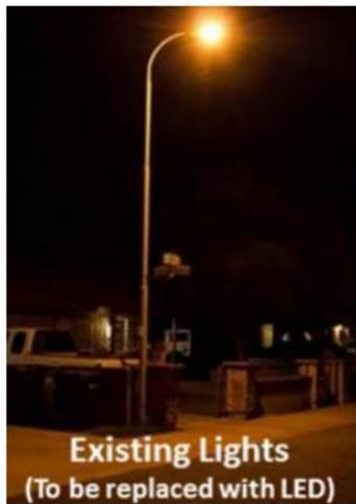
Existing 2200 Kelvin HPS
