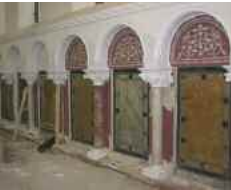
In this example, the original decorative paint scheme is being recreated based on detailed evidence
