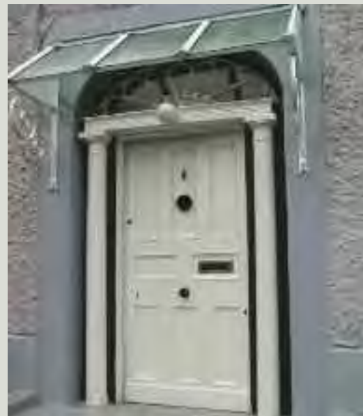
This aluminium canopy is an inappropriate addition to the early nineteenth-century doorcase. Any proposal to remove it should ascertain if the fixings have damaged any cut stonework that might survive beneath the modern render
