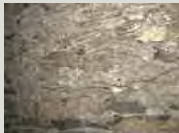
Evidence may survive on a plastered vaulted ceiling or arch of the wicker centring used in forming the vault, seen in the hollows left by the wickerwork which was embedded in the plaster and left there when the centring was removed. In some rare examples, pieces of wickerwork also survive
