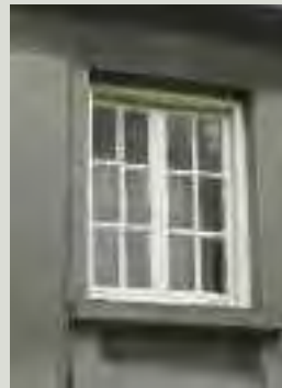
Casement windows, although widely used in many countries, were seldom used in Ireland after the arrival of the sash window in the late-seventeenth century. Eighteenth- and nineteenth-century casement windows, whether of timber or metal, generally open inwards, excepting French windows, which open out onto terraces or balconies
