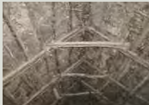
Unwrought or partially-wrought roof structures, however simple or slight they may seem, are part of the historic vernacular fabric. Repairs should aim to support the existing structural elements with new timbers rather than replace them
