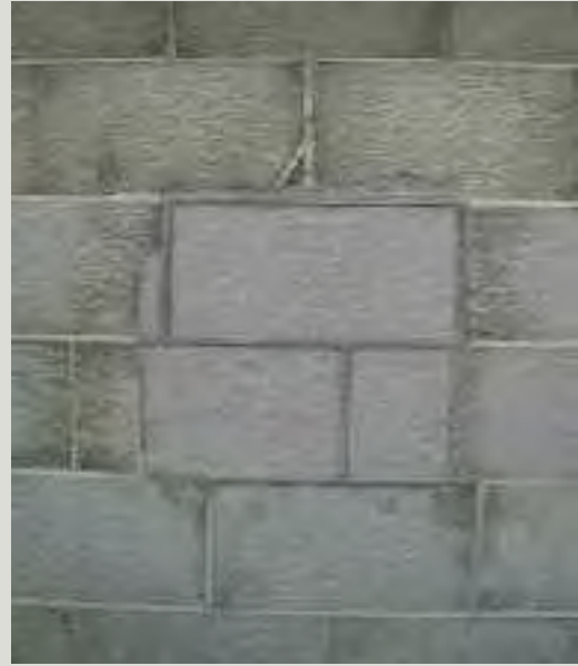
The repair of concrete structures should be carried out so as to resolve the underlying problem without a visually obtrusive result. In this illustration the repair to the reconstituted 'stone' will tone down in time although the strap repointing is inappropriate
