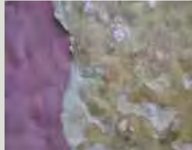
The way that limewashed render weathers contributes greatly to the patina of age: as it rubs away layers of different colours may be exposed. New coats of limewash can be applied as necessary without removing the existing layers
