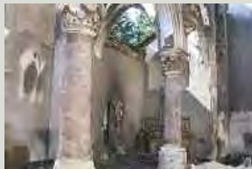
Where a protected structure has suffered devastating or irreparable damage to its special interest through a fire or other disaster, it may often serve little purpose to reconstruct or replicate it, except where a larger architectural design has been affected by the loss or the structure is an important local landmark; in such cases the reinstatement of the exterior or other elements of the structure may be considered
