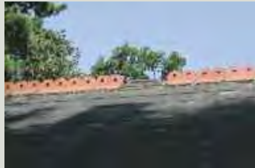
Where it is proposed to ventilate roof spaces, important architectural details should be retained intact; in this example a pierced ceramic tile has been replaced by a new vent tile which disrupts the line of the ridge comb and damages its visual integrity
