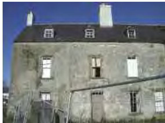
Derelict buildings can become targets of vandalism if not properly safeguarded
