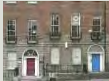
Openings that were later created or remodelled can contribute to understanding phases of the history of the structure. The late eighteenth-century fashion of lowering windowsills altered many earlier openings, but they can now be seen to represent a valid phase in the structure's history. Restoring these windows to the original proportions would require the loss of later fabric of historical interest and should only be undertaken in exceptional circumstances, based on sound evidence and after all alternatives and potential consequences have been fully explored
