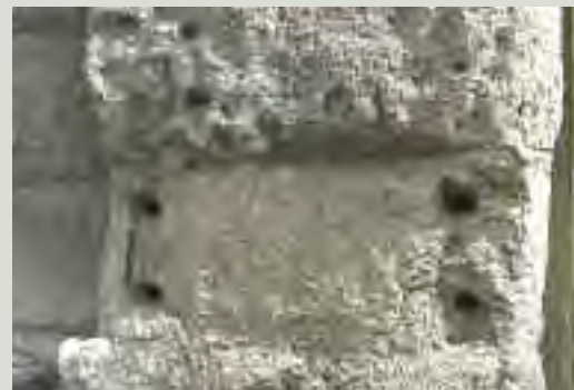
The removal of signs may cause or exacerbate existing problems. In this case rusticated masonry was cut out to recess the sign. Now that the sign has been removed, the damaging consequences of the work are all too obvious
