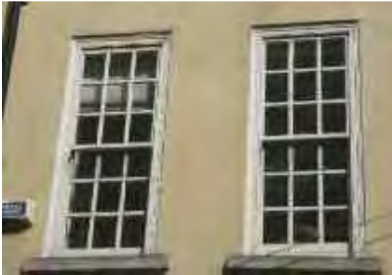
These replacement windows, although in many respects well detailed, have horns on the sashes, which is incorrect for the period of the building
