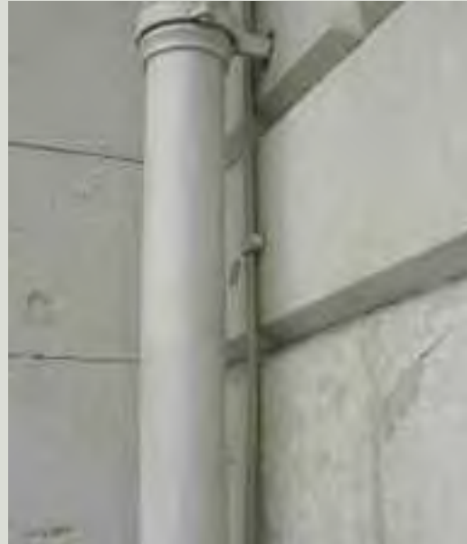
Lightning conductors may be a requirement on tall or otherwise vulnerable structures. The conductors should be channelled to earth unobtrusively; this example shows a discreetly coloured lightning conductor carefully concealed behind a downpipe
