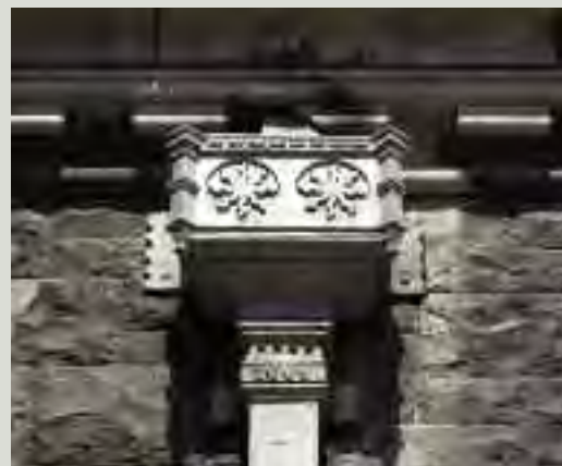
Good conservation practice encourages the honesty of repairs and alterations which may be discernible to the expert eye but not visually obtrusive. This new hopper head was designed to match the style of the structure but is recognisable, on close inspection, as a new element from its 1999 date
