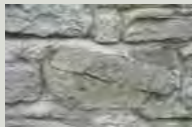
Even durable stones such as granite and limestone can be irreparably damaged by inappropriate works. The cement mortar used in repointing this wall is stronger than the stonework. As a result, structural movement in the wall could not be absorbed by the mortar and instead the stone has fractured. The impermeability of the mortar may cause future additional damage, as any water entering the wall through this fracture will be unable to escape
