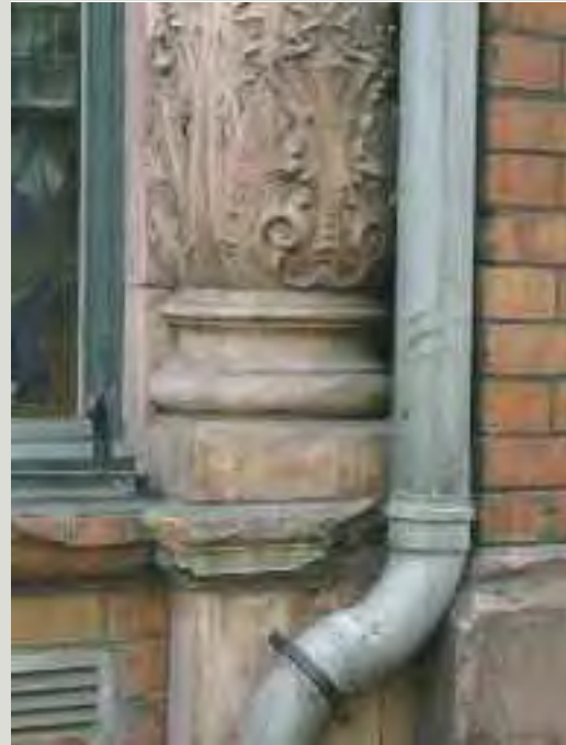
The ill-considered fixing of new items such as pipework to the principal elevations of structures can adversely affect their architectural quality and cause physical and irreversible damage, as has happened in this case where a fine architectural element has been cut through to facilitate the location of a new pipe
