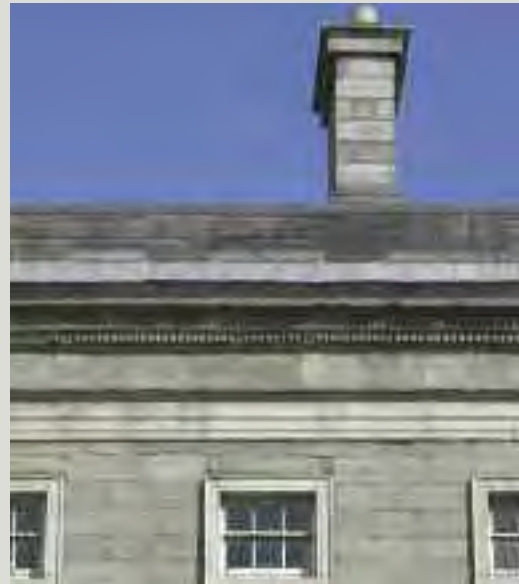
The eaves of a building can be vulnerable to weather-related problems, typically parapet walls become saturated as they are exposed on both sides to rain. Problems will also arise where the blockage of the gutter concealed behind a parapet may not be readily noticed. However, where they exist, parapet walls are usually an important architectural feature of the building
