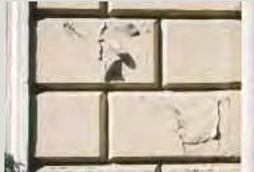
Applying impermeable paint to render or masonry can inhibit the necessary passage of moisture through the fabric. Unsuitable paints may peel off, sometimes shortly after application
