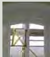
Glass is more vulnerable than most materials to damage during works, especially during the erection or dismantling of scaffolding. Historic glass should be protected at least to the exterior and, if necessary, also to the interior. Glazed windows should never be broken to facilitate scaffolding poles or ties, nor held open unless adequate protection is given to the glass and the sash is supported
