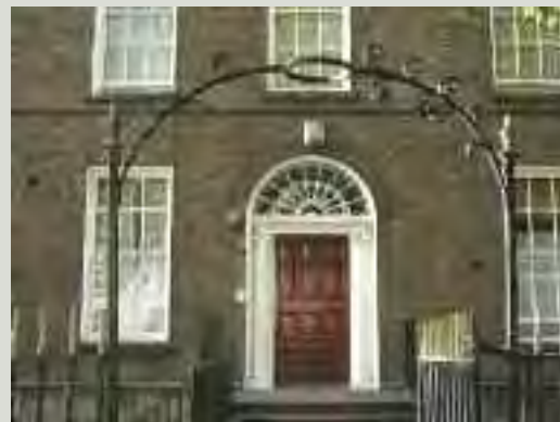
Boundary features such as gates were often designed and located to enhance the approach to a building, as seen with this example of an arched lamp bracket sited to light the gateway and path to the front door. Relocating or removing such features would not only make them liable to damage during the works but may also adversely alter the relationship between the structure and the features of its curtilage
