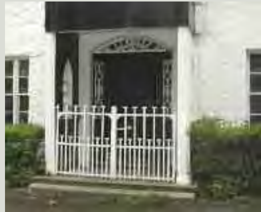
This porch has undergone at least one phase of alteration, although several elements of interest survive, such as point-arched cast-iron windows, strapwork gates and stone steps. Any proposed restoration of a porch such as this should be well detailed, based on good evidence and incorporate surviving features of interest
