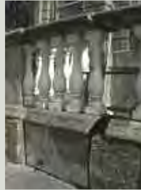
This elaborate access gate to the basement area is fabricated of plate and cast iron to match the adjacent stone balustrade. Surviving high-quality eighteenth-century iron balustrading such as this is rare and significant
