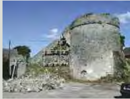
Ivy has been removed from this mediaeval mural tower after an detailed record was made of the fabric to ensure that potential loss or damage to the stonework could accurately be remedied, reusing the historic fabric without resort to conjecture
