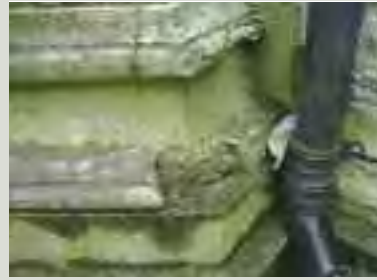
Damp problems arise more often from poor maintenance or poorly-executed repair works than from inadequate original detailing.
