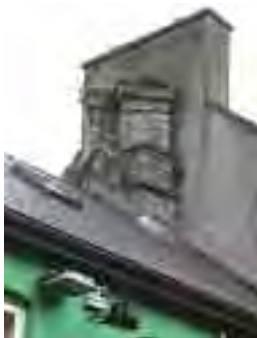
Adjoining buildings that are protected structures may be impacted upon, either directly or visually, although not actually part of the development site. This will be particularly obvious in the case of terraced buildings as in this example which has an important surviving mediaeval chimney stack on a party wall
