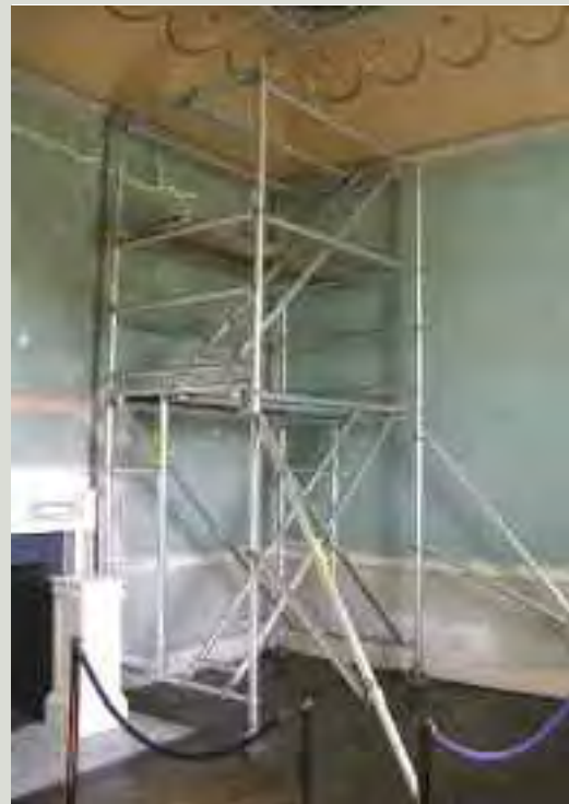
The erection and dismantling of scaffolding in rooms or spaces with important surface decoration or finishes requires especial care. Scaffolders experienced in such work may be required in these circumstances
