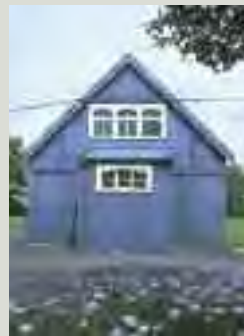
Metal sheeting consisting of flat or corrugated panels of iron, steel, lead, copper or zinc was used to clad many types of buildings, including places of worship such as this small church. Early metal sheeting is often of technical interest and should be identified and, where necessary, repaired, unless an inherent design fault requires its replacement to an improved specification
