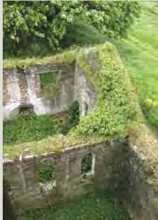
Exposed wall heads are generally the most vulnerable parts of a ruined structure. The method proposed to cap exposed wall heads should not result in water being trapped inside the core of the wall and should be visually acceptable. In some cases, the ruinous structure may need to be monitored over a period of time before a decision can be made as to what work might be appropriate
