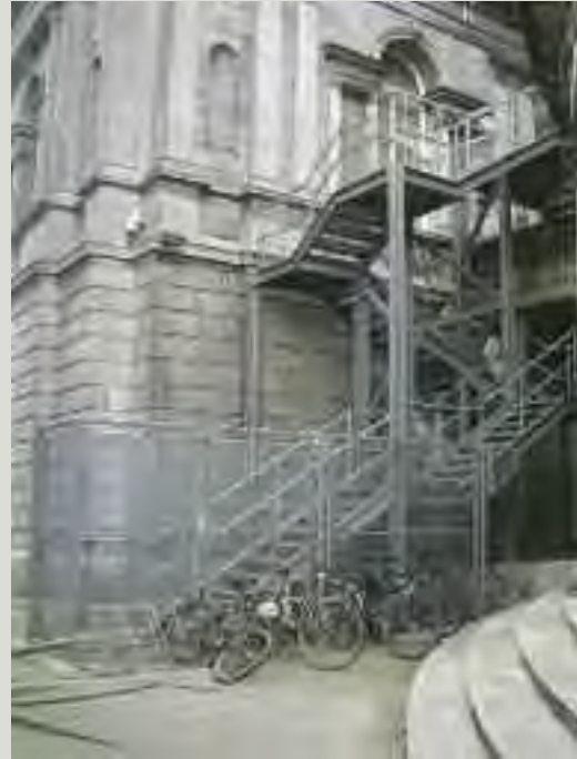
The use of external escape stairs should be avoided on important elevations or where they would be obtrusive in an important view of the structure
