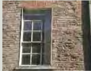
The decay of the soft handmade bricks of this façade has been accelerated by the use of extensive and poorly-executed cementitious mortar repairs coupled with strap pointing
