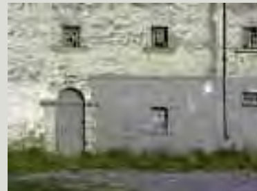
The conversion of this 1762 Charter School nursery to a store in the nineteenth century involved partially blocking the window openings, thereby altering its character. Restoring the openings would be possible using surviving evidence in the fabric and employing historically accurate detailing. This approach is appropriate where the character of an architectural composition can be restored by undoing later alterations of little interest
