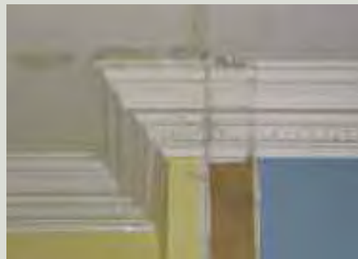
New partitions, where considered acceptable, should avoid disturbing historic fabric. They should be scribed around cornices, dado rails and skirtings to allow removal without damage. However, it is not generally recommended that important spaces within a protected structure be subdivided even if the subdivisions are reversible
