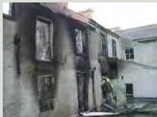
As soon as it is safe to do so, the surviving fabric of a damaged structure should be inspected and measures taken to stabilise it, erecting a temporary roof if necessary and securing the site against unauthorised access
