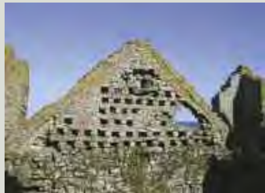
Some ruins may require careful dismantling and re-erection of parts of walls that have become unstable. In this case, apart from the repair work required to the gable (containing pigeon nesting boxes), it is intended to re-roof the building. Where it is appropriate to re-roof a ruinous structure, the aim should be to retain the maximum amount of original fabric
