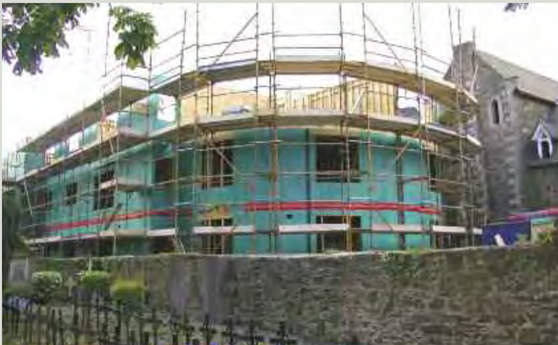
New development in the grounds of this important Gothic revival former convent is under construction between the structure and the nuns' graveyard and has altered their historical relationship
