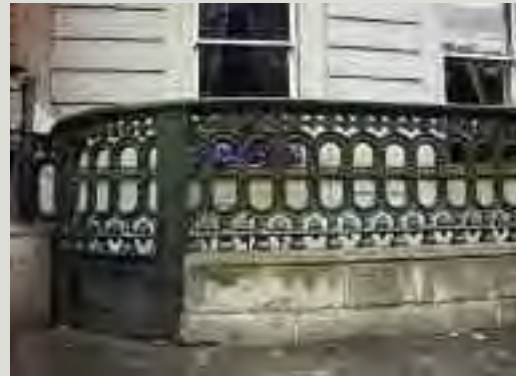
The careful repair of a damaged feature such as a cast iron balustrade contributes much to preserving the character of a structure (shown here before and after repair). Where elements are not capable of repair, the new work should accurately reproduce the detail of the original. Entire sections should not be replaced if only a part is damaged
