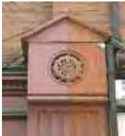
The application, and subsequent removal, of paint from terracotta (and soft stones such as sandstone) can cause damage to the material and jeopardise its future conservation
