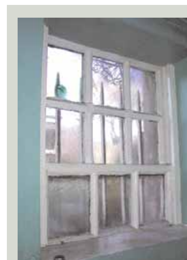
Condensation problems are best solved by reducing the moisture level of the air inside the building. While a dehumidifier may be useful for coping with the aftermath of an individual flood, the only successful long-term solution is to improve the levels of ventilation
