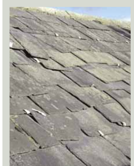
A number of tingles have been used in previous repairs of this roof but the slipping of slates continues, indicating a widespread failure of fixings. As a rule of thumb, where a third or more of slates have slipped the entire roof will require to be stripped and re-fixed, reusing the existing slates where possible
