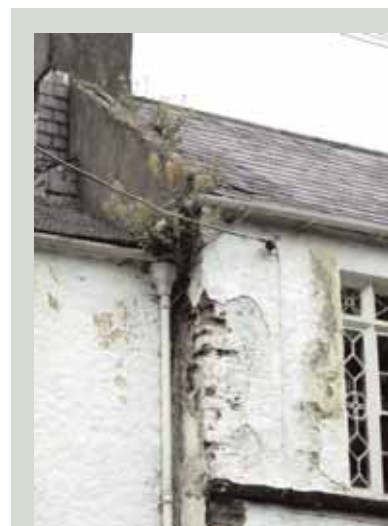
Damp problems in ground floor or basement rooms may not be caused by rising damp but by rainwater from broken gutters above saturating the wall and the ground beneath
