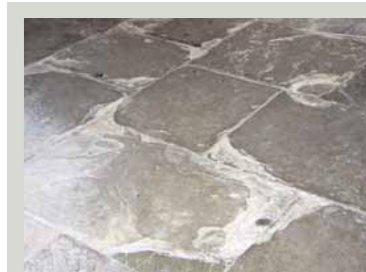
Stone flags in basements were often laid directly on the earth below. It is essential that their surfaces are not sealed or the joints between flags filled with cement as this will trap moisture in the stone and cause decay
