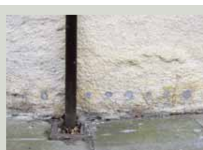
The drill holes associated with injecting a chemical DPC can be unsightly. A more effective method of dealing with the damp problem in this case would have been to reduce the level of the impermeable paving around the building and ensure that rainwater drains away from the base of the wall
