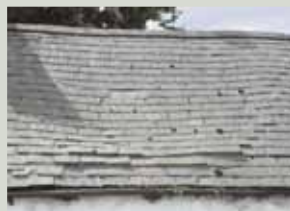
This roof is showing signs of sagging which probably indicates decay or damage of the structure beneath which must not be ignored
