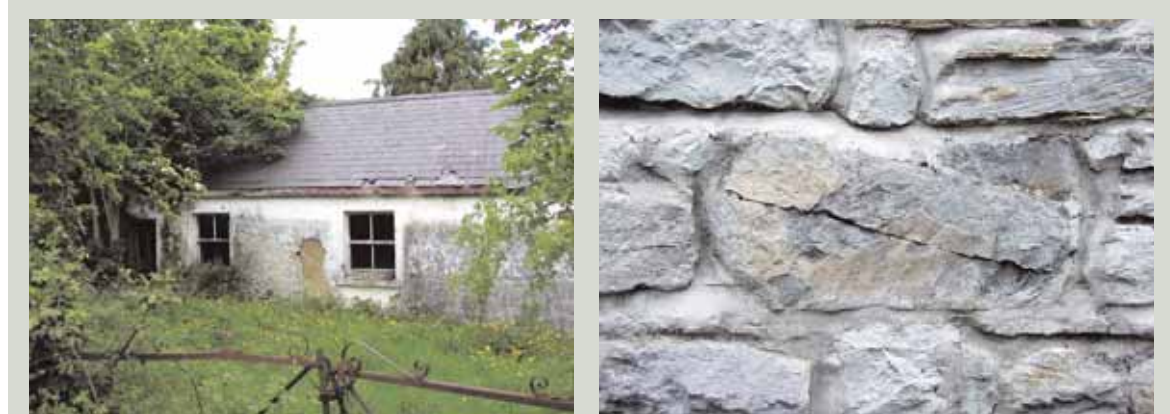
Traditionally-built buildings need to 'breathe', allowing the moisture absorbed during wet conditions to evaporate when the weather is dry. Inhibiting this process by letting trees and other plants to grow up close around a building or using the incorrect materials in repair can cause decay to set in
