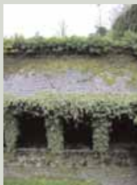
All plants growing against external walls should be clipped back regularly to avoid blocking gutters and concealing defects in the wall behind
