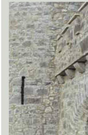
Dealing with structural cracking in walls requires specialist advice. Cracks can be successfully repaired once the cause of the structural movement has been identified and the problem solved
