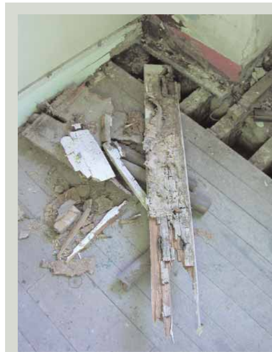
Timber which has suffered dry rot attack has a distinctive cuboidal pattern of cracking. Only timber which has decayed to the extent that it can no longer do its job should be removed in the course of treatment
