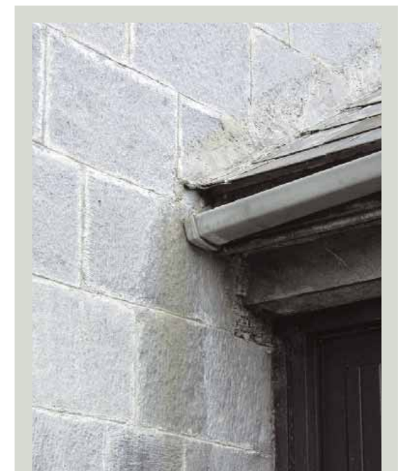
The end of this replacement gutter has not been properly fixed and has begun to sag with the weight of water trapped in it. Already the wall has been stained and there may be further damage if the saturation continues
