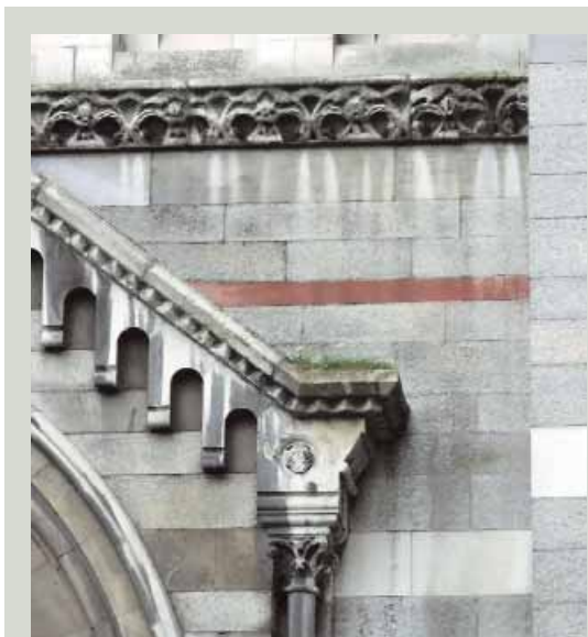
Parts of a building may be difficult to access and are likely to be neglected for that reason. Plants have begun to take root on this high level decorative detail and should be removed before they cause damage to the fine stonework
