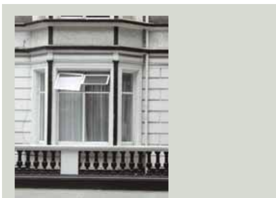
Well-maintained and repaired historic windows can last for hundreds of years. Unfortunately they are often needlessly replaced with poor-quality modern windows which soon fail and require renewal
