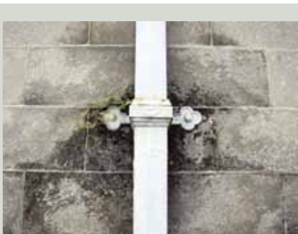
The staining of the stone wall behind this downpipe joint suggests there is a blockage inside the pipe. If the water trapped inside freezes in cold weather, it may burst the pipe
