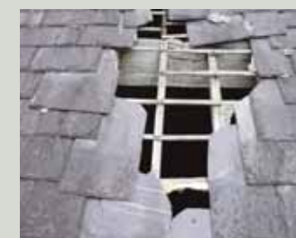
Slipped or missing slates must be attended to as a matter of urgency before damage is done by penetrating rainwater
