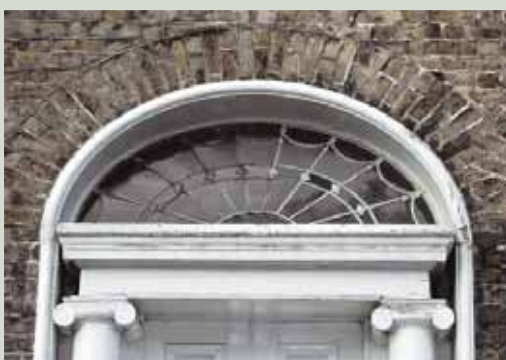
The cleaning and repair of fanlights is a delicate task which should be left to a specialist
