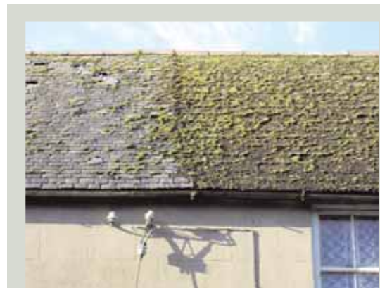
Moss growth is likely to take hold on more porous cladding materials such as clay or fibre cement tiles. It must be regularly removed from all roof types as it can force open joints between slates and tiles allowing water into the roof space
