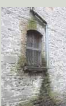
Leaking joints and missing sections of downpipe are relatively cheap and easy to fix if attended to promptly. When defects are not remedied, they lead to serious problems which are expensive to repair and involve the loss and disruption of parts of the building fabric
