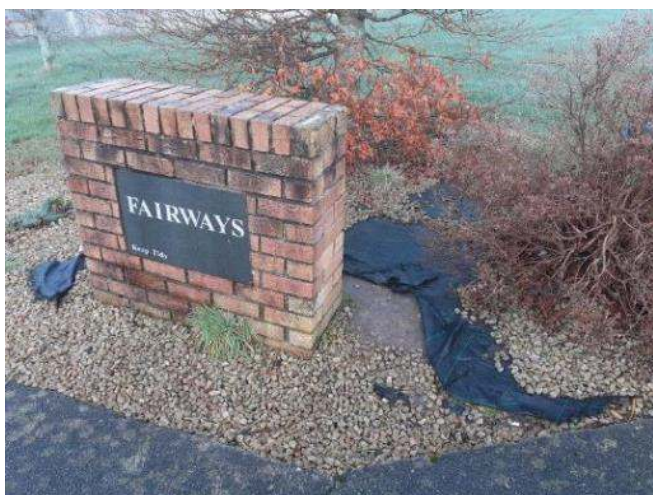
Plate 54: In this case the weed-prevention fabric has become exposed beneath the gravel
