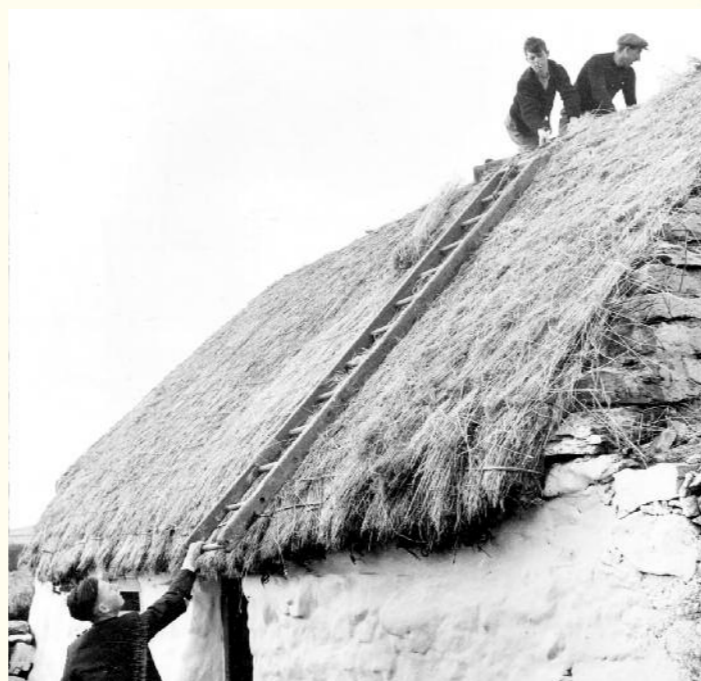
Thatching a roof on a cottage in the West of Ireland in 1950.
