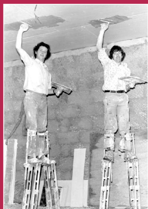
Construction of a new stand at St Tiernan's Park, Crossmolina, in 1978. Picture: Western People Archive
