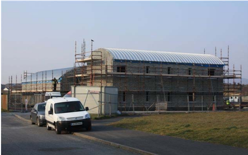
On-going works on the new Quay Community Centre, for Westport Town Council
