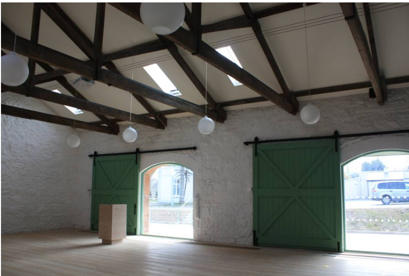
Interior view of the newly refurbished 'Railway Goods Shed' and the beautiful kingpost trusses visible in the interior of the space - now to be used as a Cultural & Community Centre
