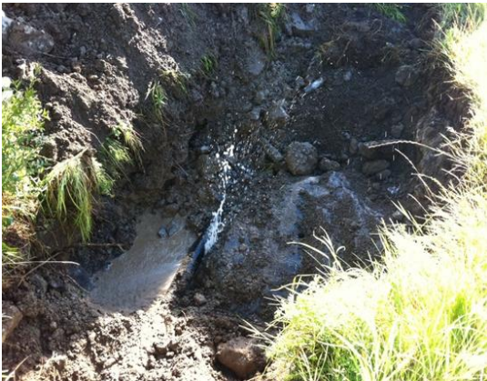
Fig 3: 120m³/day leak on 75mm mains
