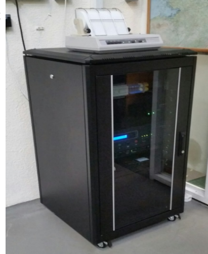
New Communication Equipment
