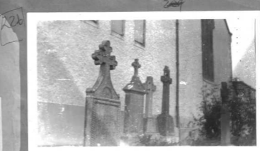
TOMBSTONES REMOVED FROM SIDE TO GABLE DURING RECONSTRUCTION WORK. Photo. taken Nov. 1st, 1938.
