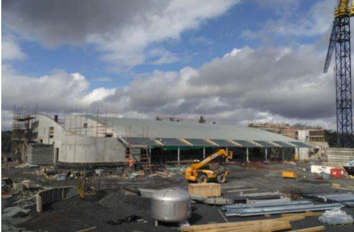
Above and below are progress photos of works to date on site.
