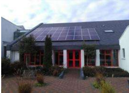
Photo Voltaic Panel Installation on the Library HQ in Castlebar.
