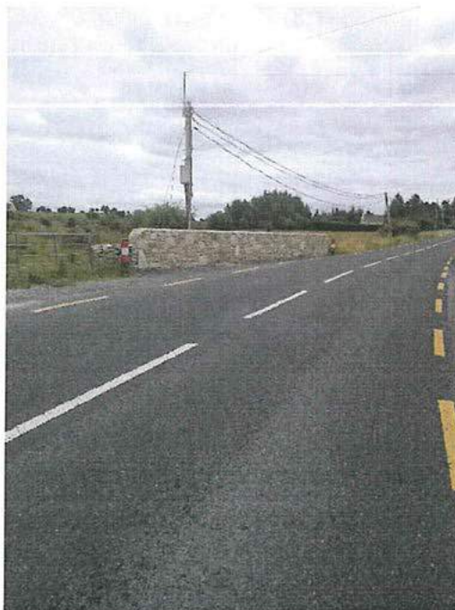
New parapet wall on Bridge on the R375 Kilkelly Rd, funded from the 2017 roads programme.
