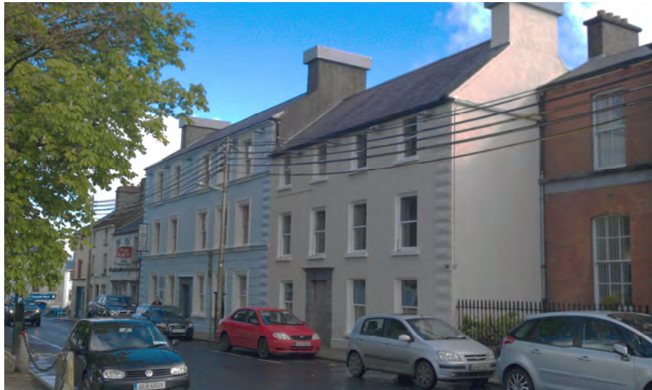
Grant approval was received with respect to The Imperial Hotel , Castlebar under the Structures at Risk Fund 2011 for essential roof repairs and associated works.
