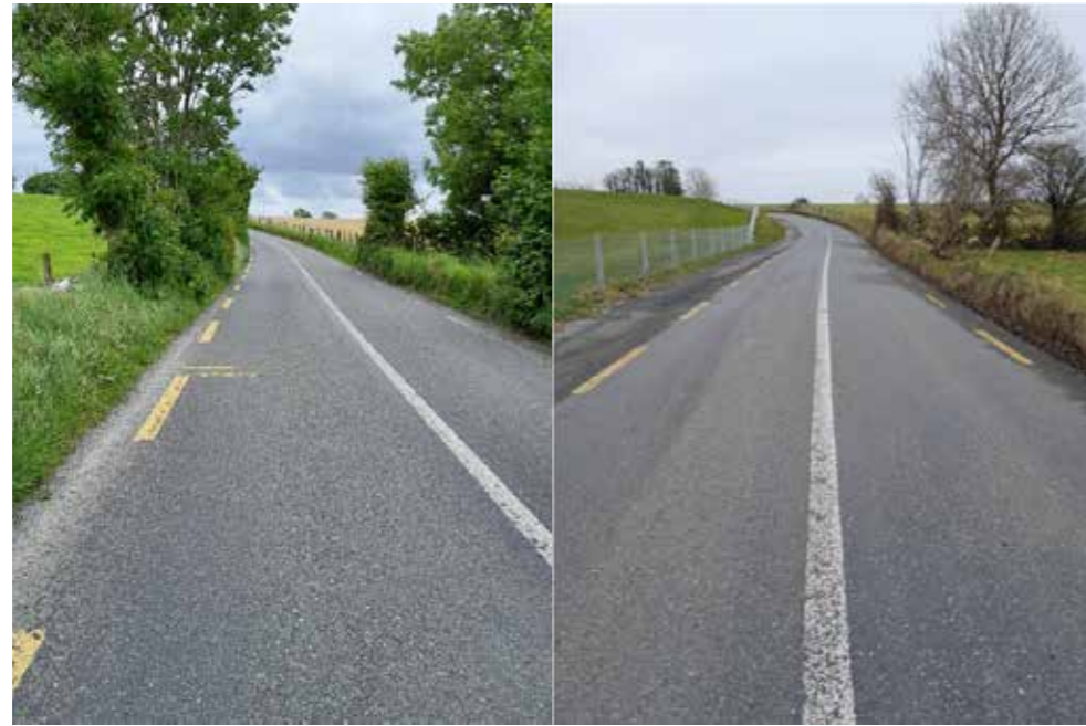
R324 Safety Improvement at Ballyrouke, Balla before works commenced and after works were completed.
