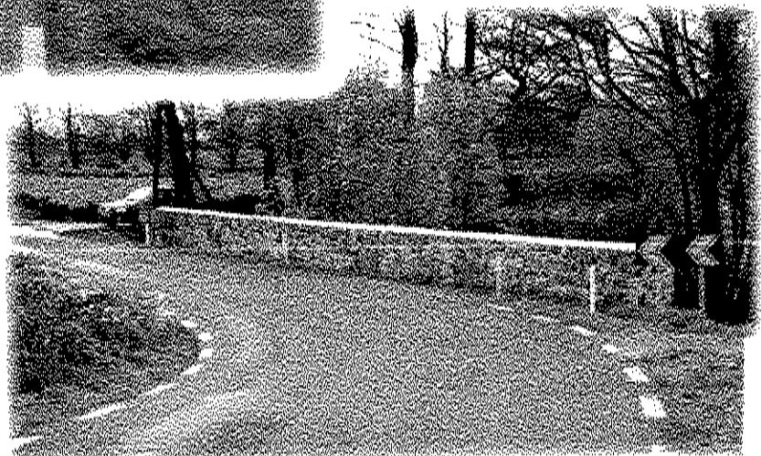
Remedial Works at Kilglassan, which included raising of existing pavement and the building of a replacement parapet wall
